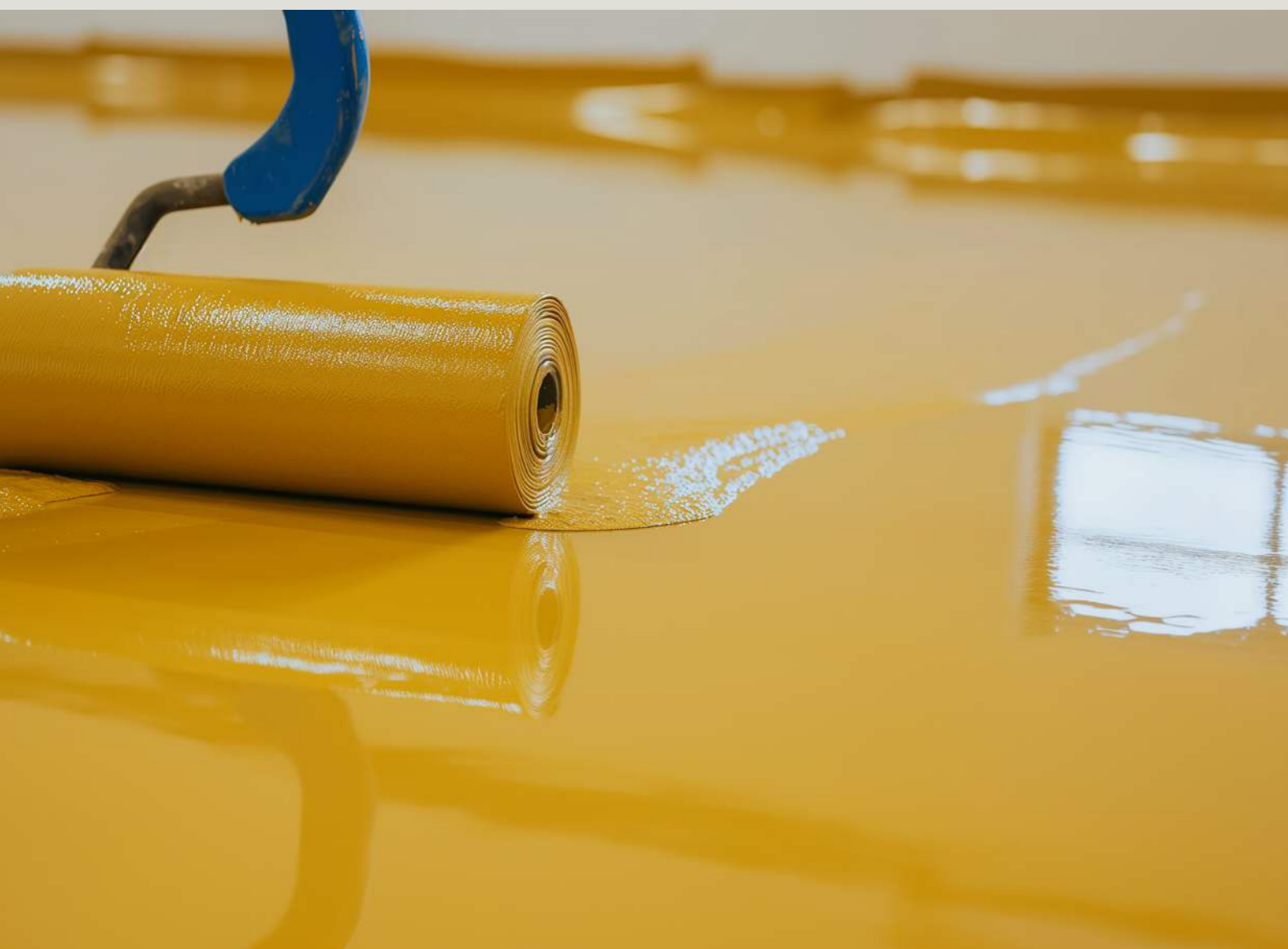
Fig. 42 Epoxy flooring. Image generated with Midjourney 6.0
